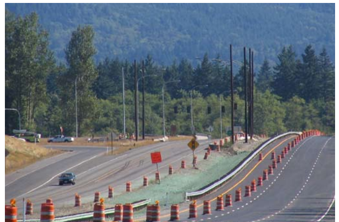
Crews turn off the signal at 244th SE - the last signal on SR 18 between I-5 and I-90.
